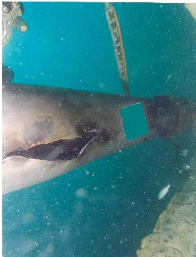
Figure 6 - Field Joint No. 451 from ZK168
