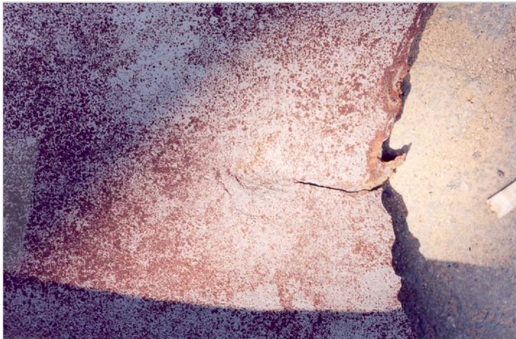
Figure 17 - Failed Joints recovered with Leak Clamp
