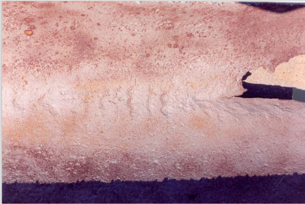
Figure 16 - Failed Joints recovered with Leak Clamp
