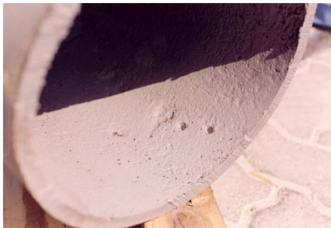
Figure 12 - Riser Tubeturn Oxygen Induced Corrosion & SRB Pits at 6 o'clock position
