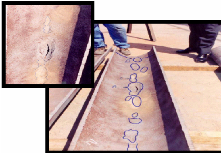
Figure 5 – Inside of the Failed Pipe Note the interconnected pits
