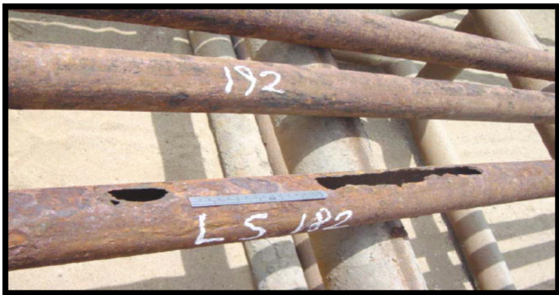
Figure 11 – Interconnected Corrosion Holes all Aligned to One Side in Contact with the Casing
