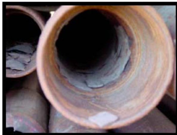
Figure 14 – Iron Oxides & Calcium Carbonate Scale Deposition on the Internal Tubing Surface of ZK-152
